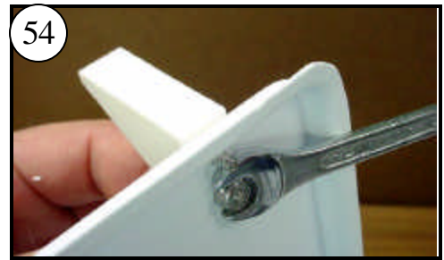
54 Attach the Tow Knees with the stainless steel nylon locknuts. Tighten with a 5/16" wrench. If they are not square to the front of the deck, adjust the holes with your drill.
